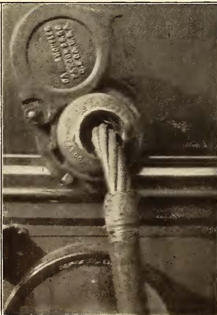
FIG. 4.—JUMPER TERMINAL WITH WIRE EXPOSED
